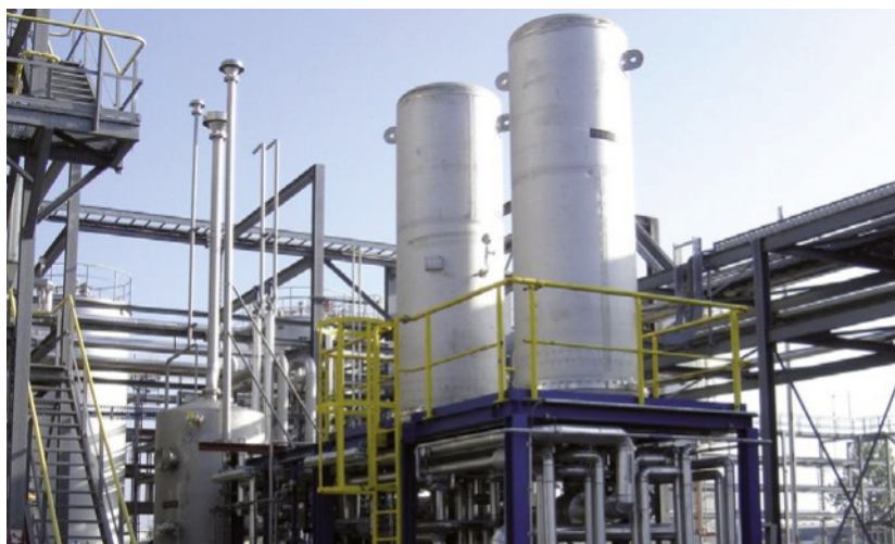
Skid mounted with membrane plant
