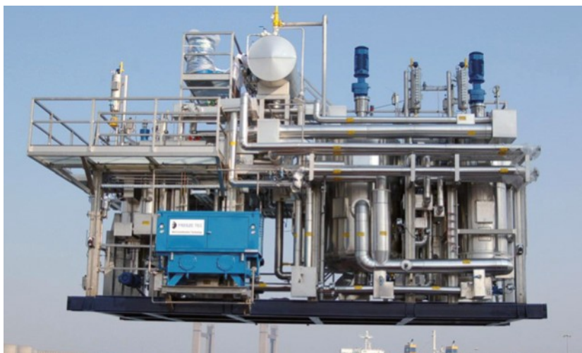
Skid mounted suspension crystallization plant for MDI
